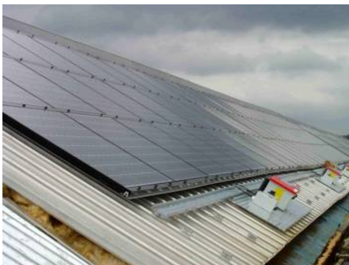
PV on the roof of Titanic Mill
